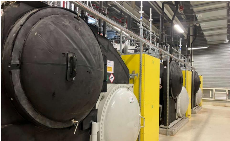
Chilled water system (condensers and evaporators)
